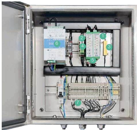
Master unit at the SCADA side
